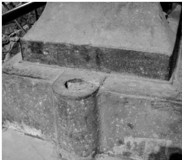
Cut mounting bolt on Pelton wheel base, Credit Author
